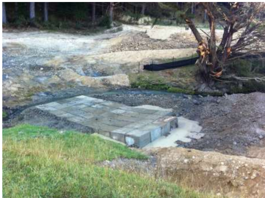
This concrete block based stream crossing (in construction) provided a cost-effective and environmentally responsible access solution at Toomey forest, Wellington Region.
